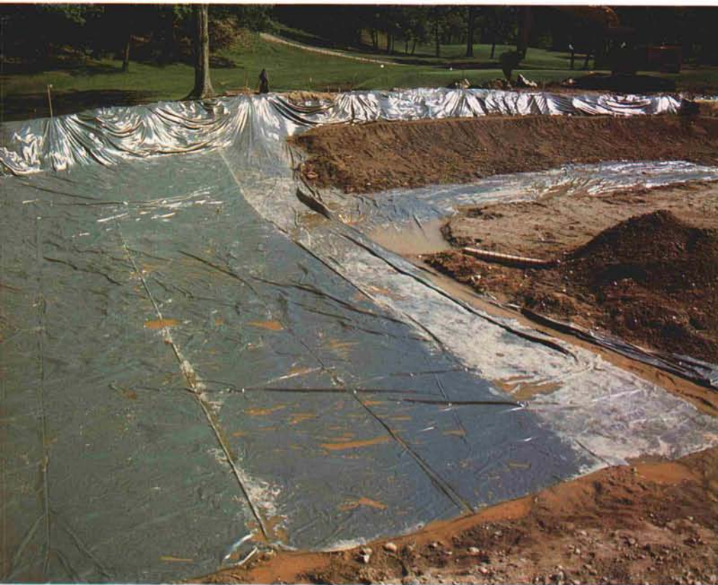
Construction of a new pond at the Brae Burn C.C., West Newton, Massachusetts.
